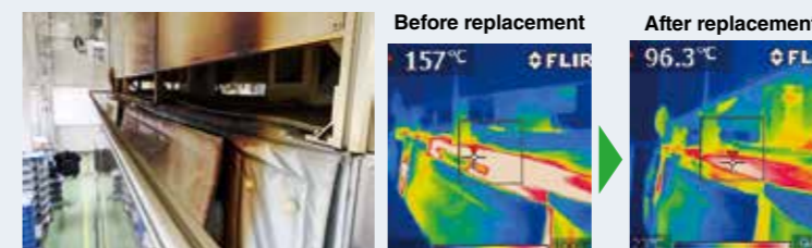
Electric heater area
